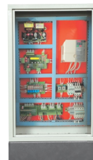
Control Panel With VVVF Drive
